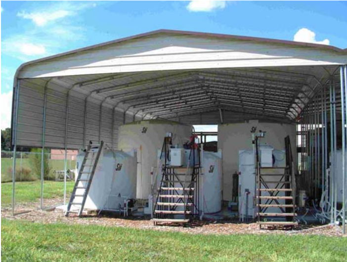
Figure 1 Process Water Tanks
